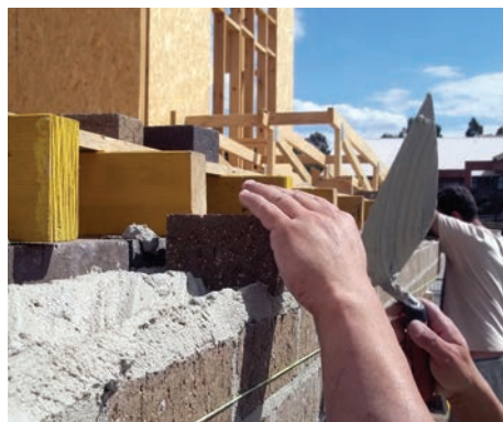
Brickwork Above Garage Door
