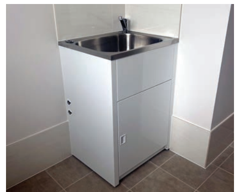
40Lt Freestanding Laundry Tub Cabinet, Ceramic Floor Tiles, Skirting Tile & Splashback Over Tub
